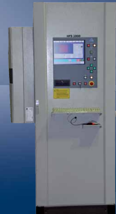
Fig.: HFS 2000 Operator panel
